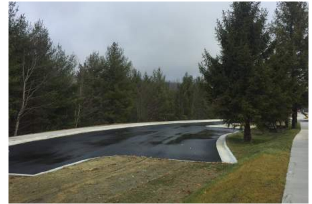
Trailhead and parking established, connecting Shoppes on the Parkway and Roots Restaurant to downtown Blowing Rock.
